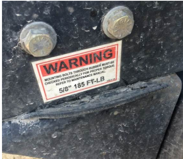
Figure 40 Isolators with excessive "push out" should be replaced.
