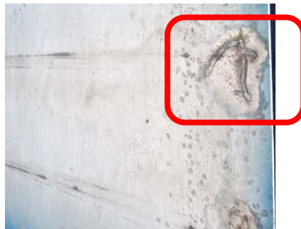
Figure 55 Roof mount system cover showing evidence of rubbing against cylinders. When repairing holes or cuts with weld beads, make sure to grind the surface smooth to reduce effects of rubbing on cylinders.
