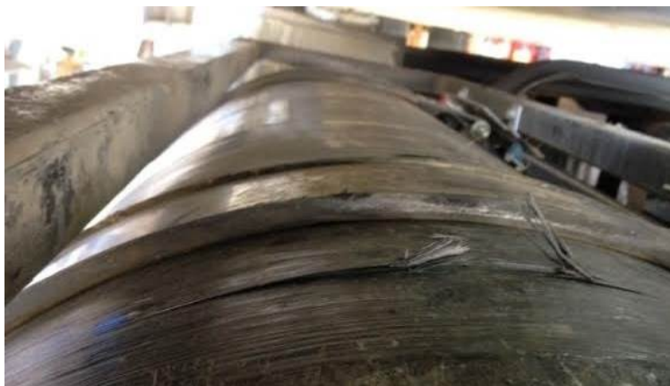
Figure 30 An example of de-bonding and delamination.
