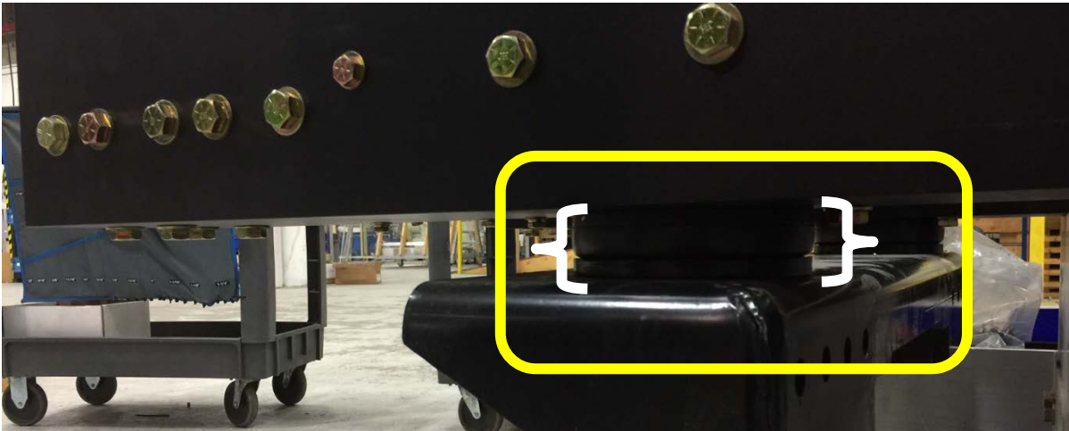
Figure 45 Measure gap between the system mounting bracket and the lower frame at each isolator and compare the differences. See text for more inspection details.
