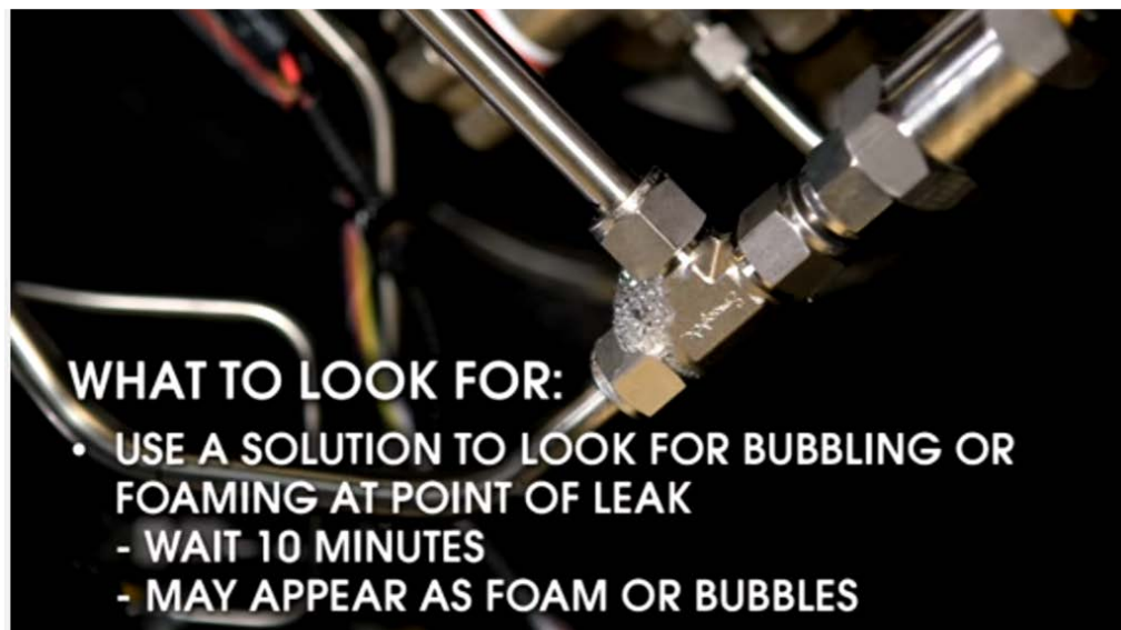
Figure 61 If you smell gas, locate leaks using leak detection solution.
