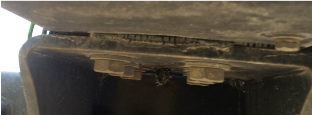
Figure 43 Cracked isolators should be replaced.
