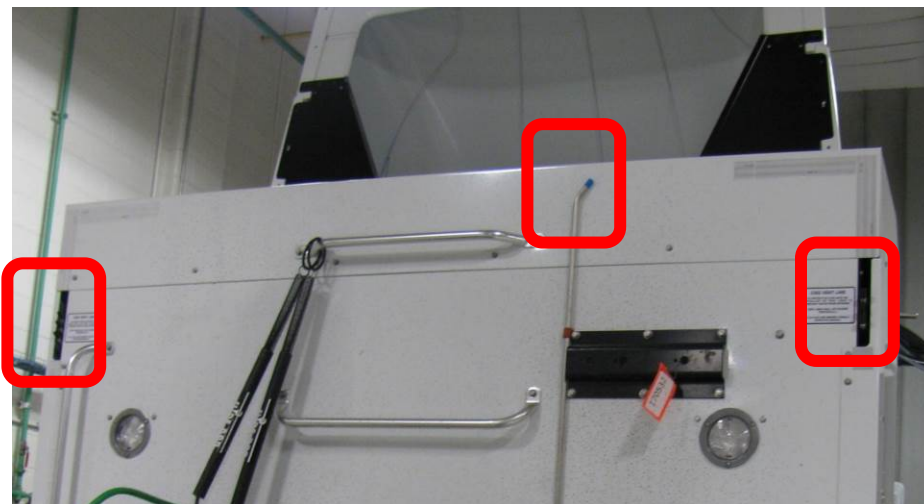
Figure 26 PRD vent caps must be in place at all times to prevent water and debris from entering the system.
