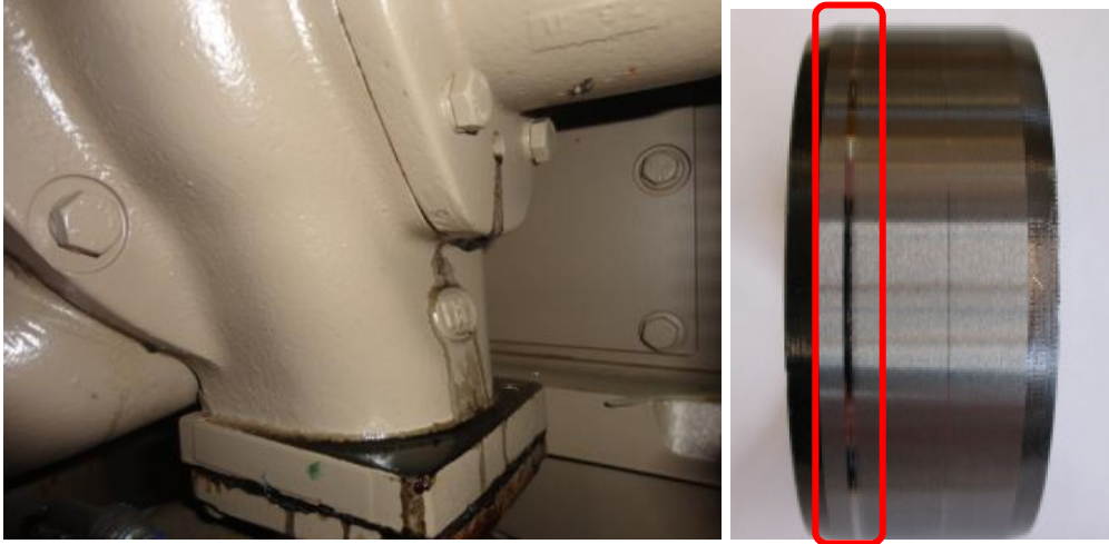
Figure 1 – example of blocked weep hole and grooved shaft / failed seal.
